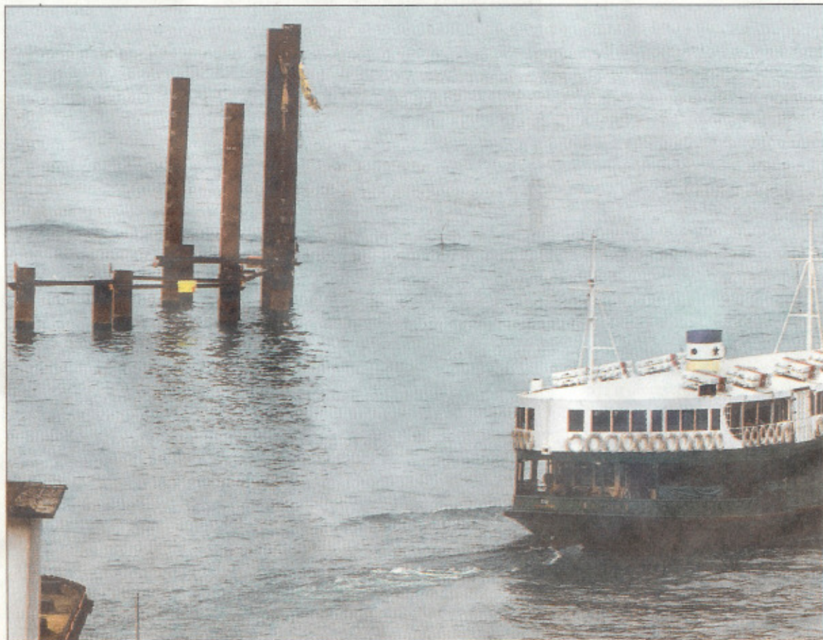
Piling works to the left of a Star Ferry in Victoria Harbour mark the start of the controversial reclamation project. AFP
